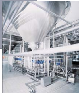
Common valve matrix installation in a tank cellar
