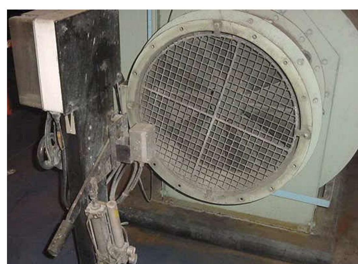
Mechanical damper systems
