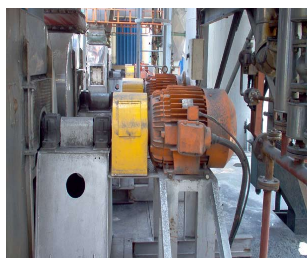
The induced draft fan is keeping the right temperature/pressure in the boiler
